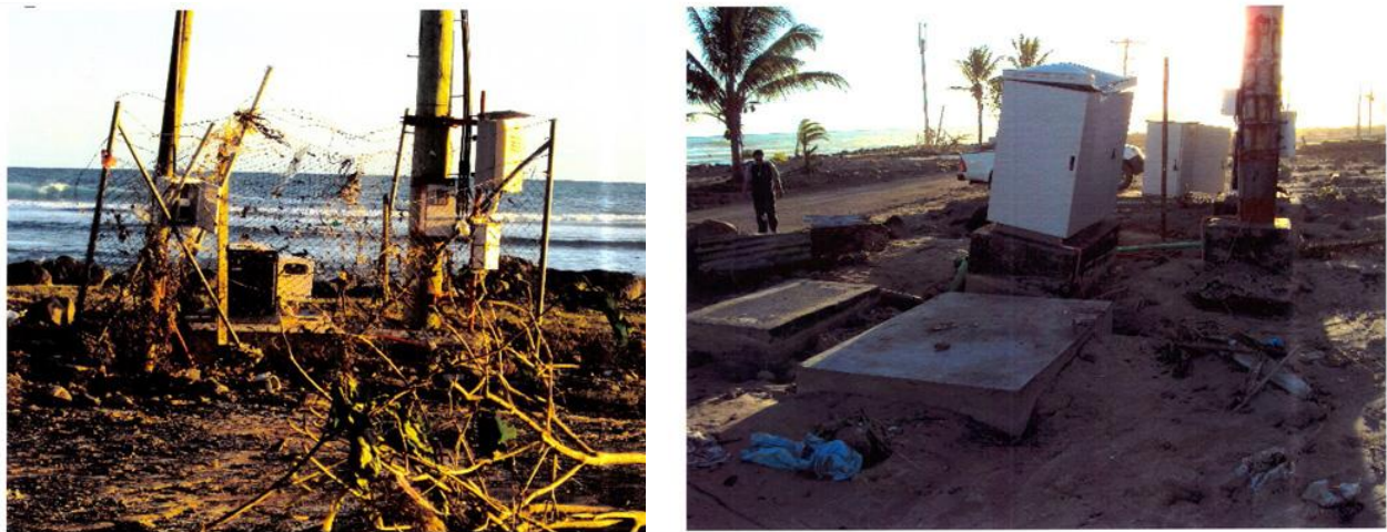
Figure 15 Damaged telecommunications sites
